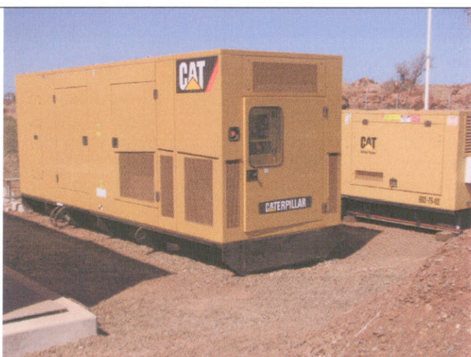
Plate 20. Internally bunded generators minimise any spills associated with machinery malfunction.
