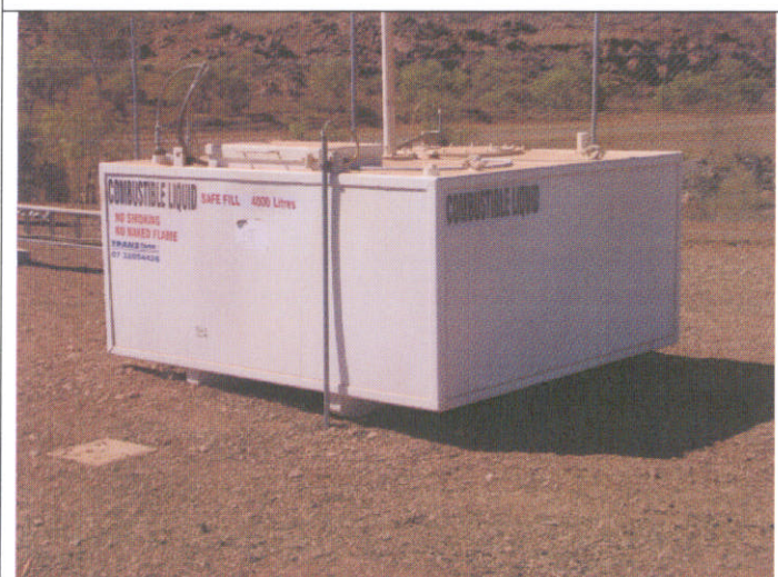
Plate 19. Diesel stored in a bunded tank with a separate bunded refuelling compartment to prevent refuelling spills.
