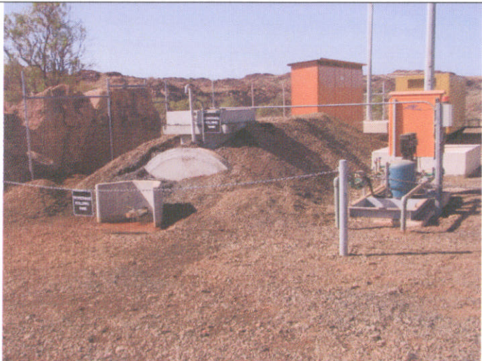
Plate 15. Site A sewage detention tank and associated level detection alarm.
